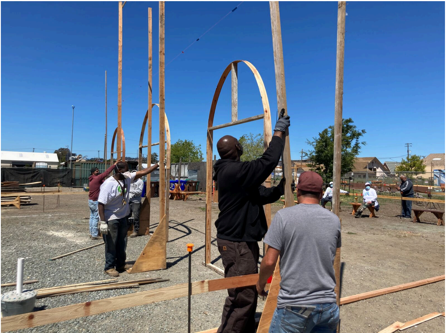
Members of the Pogo Park team, many of which are neighborhood residents who've been trained in construction and other building skills, are seen assembling the framing for Harbour Hall's distinct arched windows. Courtesy of Pogo Park
